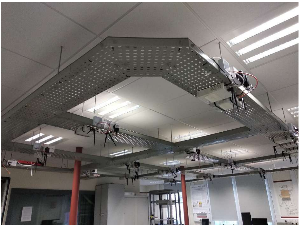
Figure 1 IRIS testbed ceiling USRP grid.
